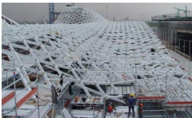
Figure 24. Structural grid during assembly (Design, Analysis and Construction of space Structure, the Mero Legacy)
