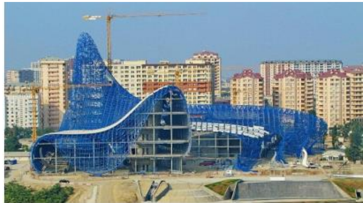
Figure 14. Cultural Center in Baku, Mero-System (Design, Analysis and Construction of space Structure, the Mero Legacy)
